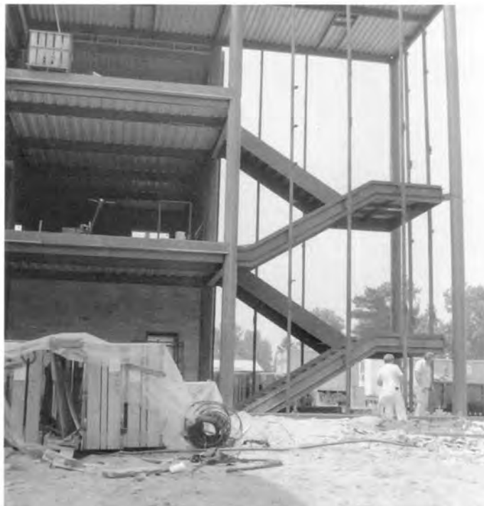
The steelwork shows the structured design of the north stair tower of the Agricultural Engineering Sciences Building during construction in 1981.
